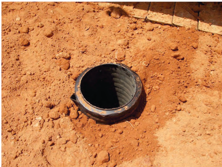
Figure 10 Jetton St. 15" diameter monitoring well
