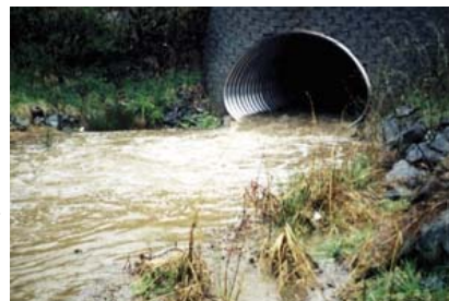
Culvert outlets with submerged tailwater conditions typically exhibit a variation in designed pool geometry from their counterparts with free-falling jets or supported jets.
